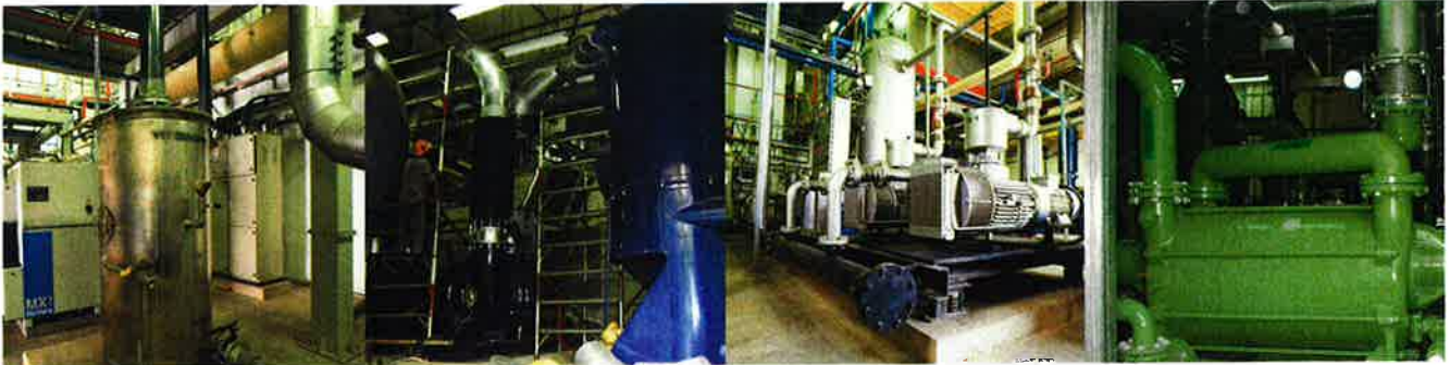
Central Wet Separator For Wet & Dry House Vacuum Cleaning System - 2x40Hp (Completed 1997)
