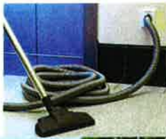
Vacuum Cleaning Inlet installed at Lift Lobby
