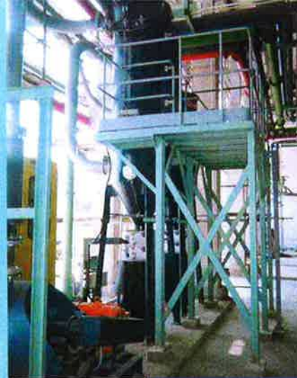
3x Vacuum Pick-up System for Waste/ Dirt Conveying, incinerating plant via Mitsubishi Heavy Industries Ltd (Completed 1999)
