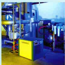
compressed air system
